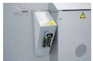
Plug socket on the furnace for the cable connection to the switchgear and control box
