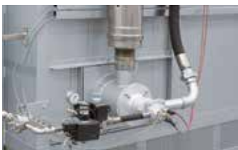
Gas burner positioned along the furnace side
